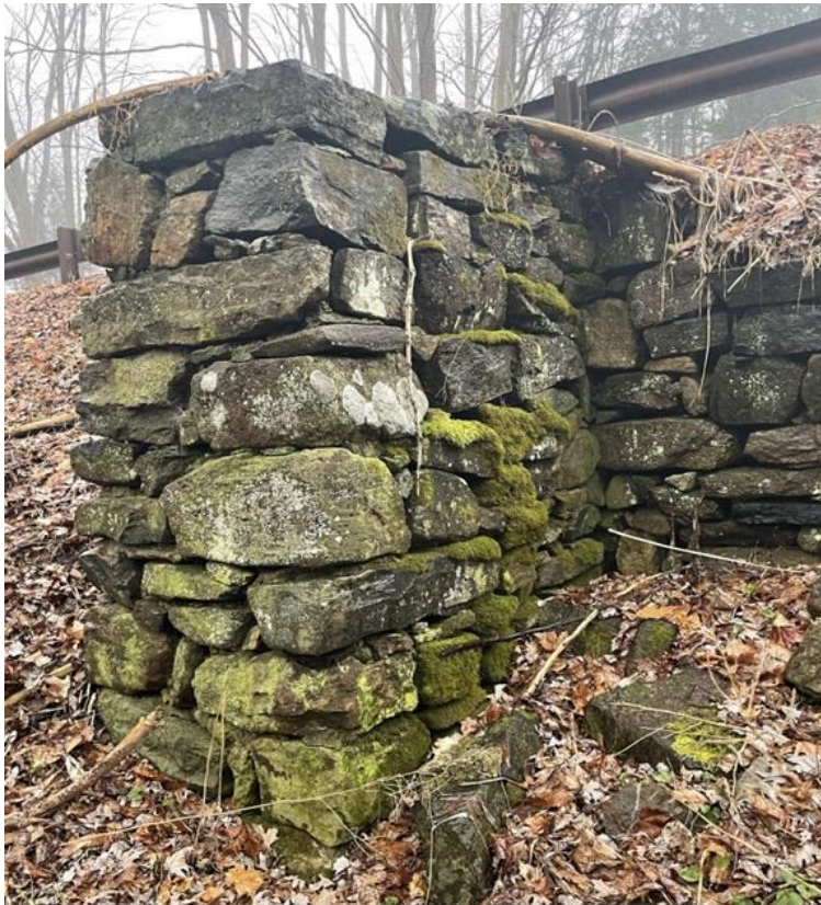
A stone foundation at the Shoddy Mill ruins alongside State Park Road.
